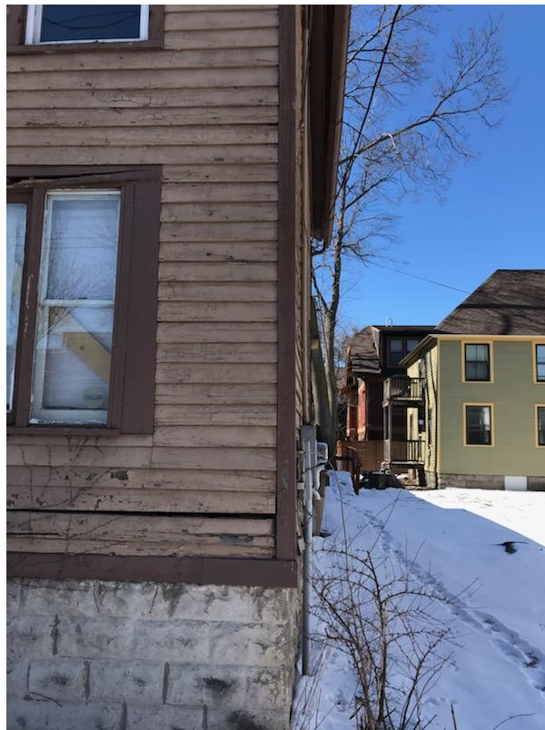
The north corner of the building is not fully vertical. Photo by Kurt Stege.
