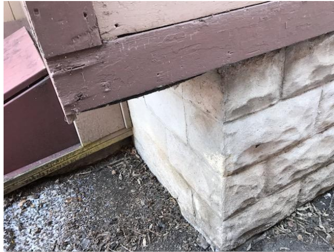
An addition on the southeast side of the home is cantilevered rather than placed directly over the foundation. Photo by Kurt Stege.
