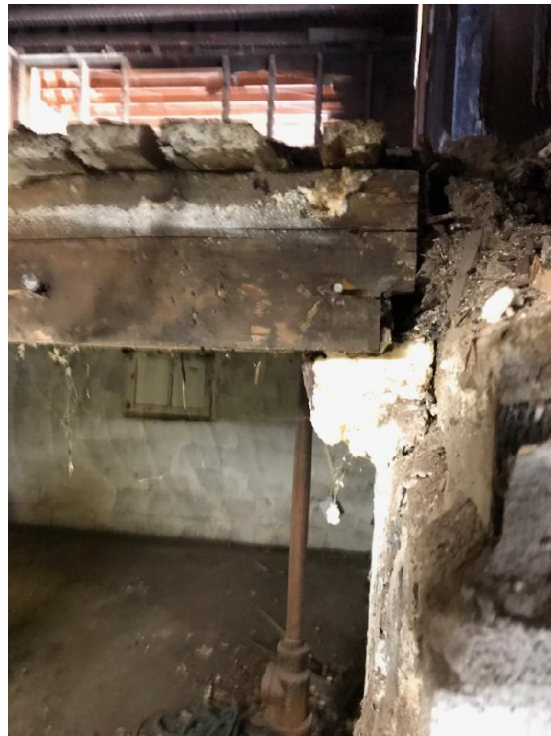
A key horizontal supporting beam for the first floor that should be resting on the foundation was never connected to the foundation and has suffered extensive rot. Photo by Kurt Stege.
